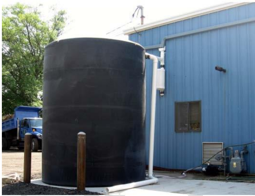
Figure 8b: A 5,000 gallon cistern used to disconnect the rooftop of the Department of Public Works in Clark Township to harvest rainwater for nonprofit car wash events
